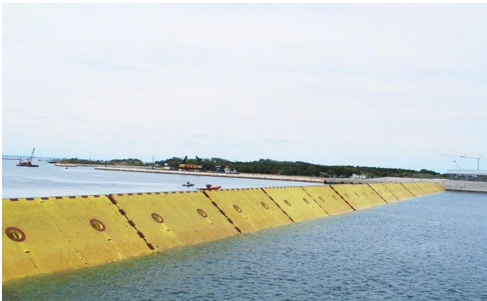
Figure 7: MOSE barrier system (MOSE, 2025)
